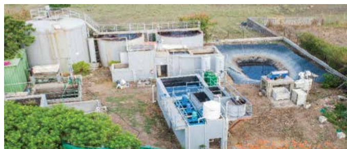
EFFULENT TREATMENT PLANT AT SULA'S NASHIK FACILITY
